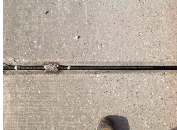
seals between deck panels missing
