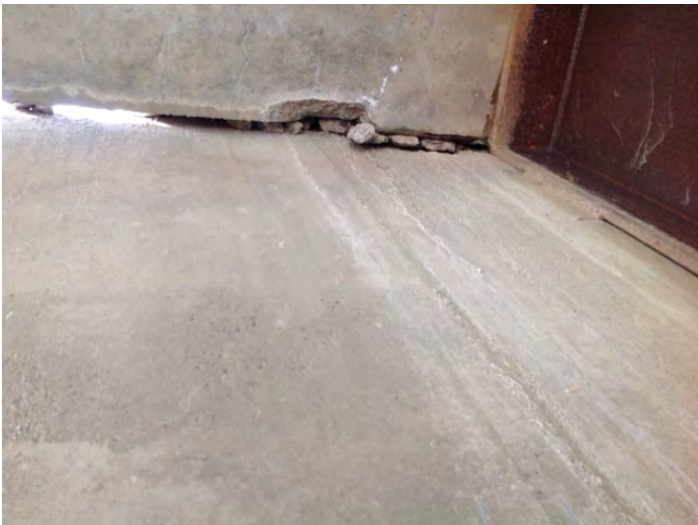
damaged deck panel
