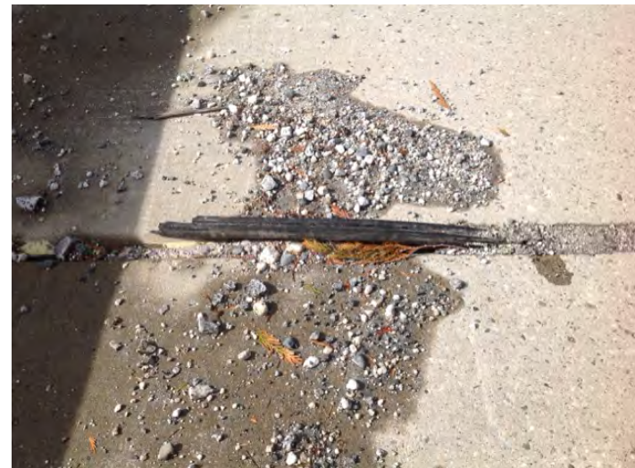
seal pushed out
