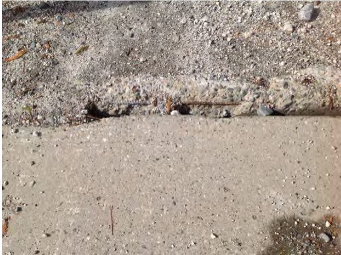
ballast wall damage
