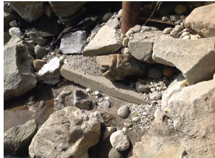
right bank - downstream footing exposed
